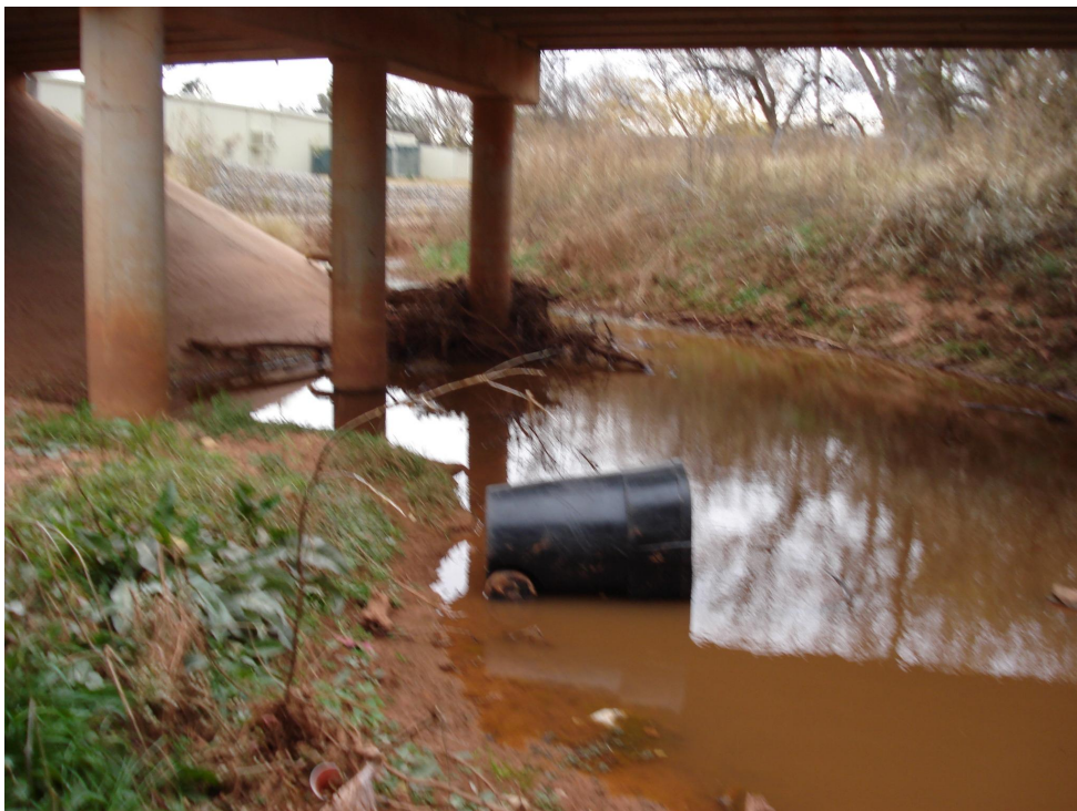
Standing water and debris in Elm Creek at Winters Freeway - north. (January 2009)
