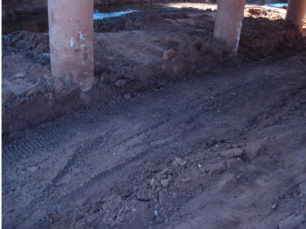
Debris and silt removed from under bridge to remove standing water. (February 2009)
