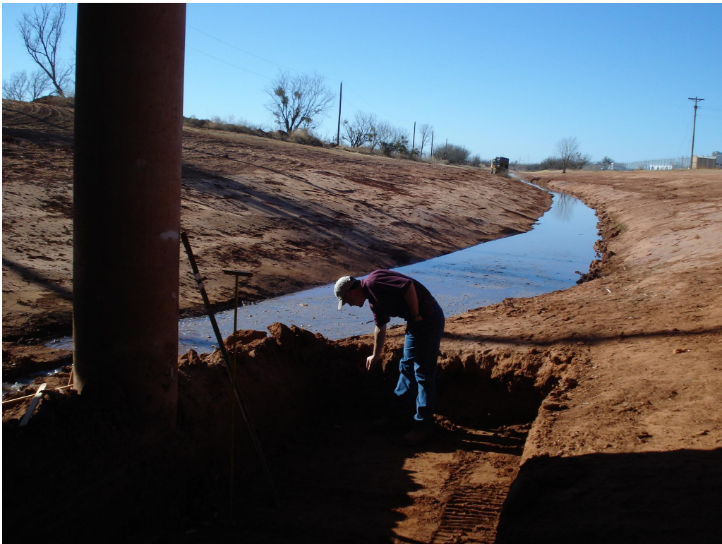
Stormwater preparing to remove final silt to release water standing on east side of Winters Freeway Bridge. Approximately 2 feet of silt removed. (February 2009)
