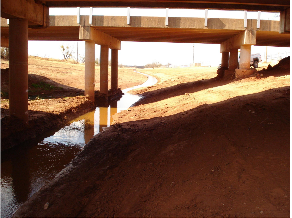
Water flowing through previously blocked drainage way under north Winters Freeway Bridge. (March 2009)
