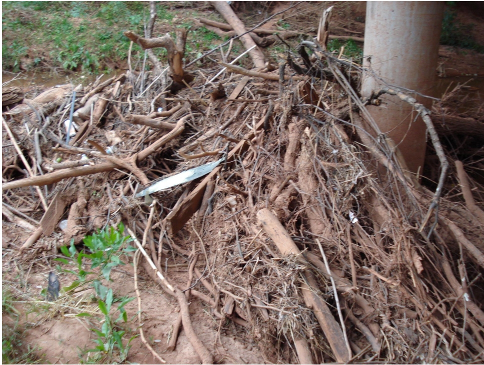
Debris accumulation in Elm Creek at Winters Freeway - north. (January 2009)
