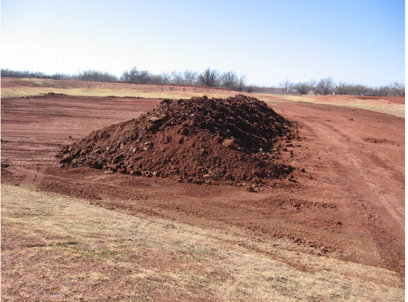
Initial stockpile of sediment to be removed. Several additional cuts were performed later to get the detention pond back to original specifications.
